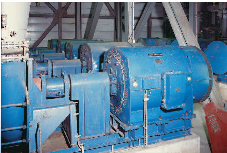
Blower drives 1,500 kW 6.6 kV 4pole, in a power station
