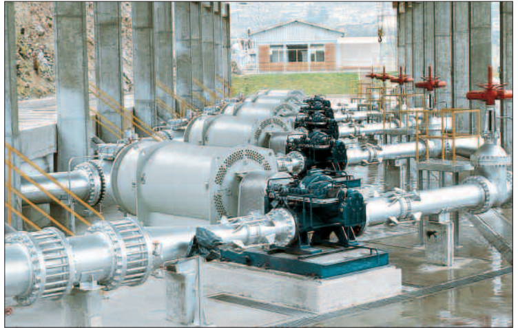
Pump drives 1,200 kW 6.6 kV 2pole, in a drinking-water supply
